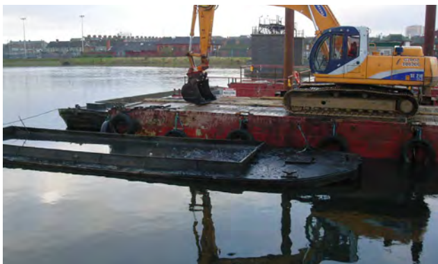
Photo 58 Dredging is an essential component of maintaining a safe and navigable waterway
