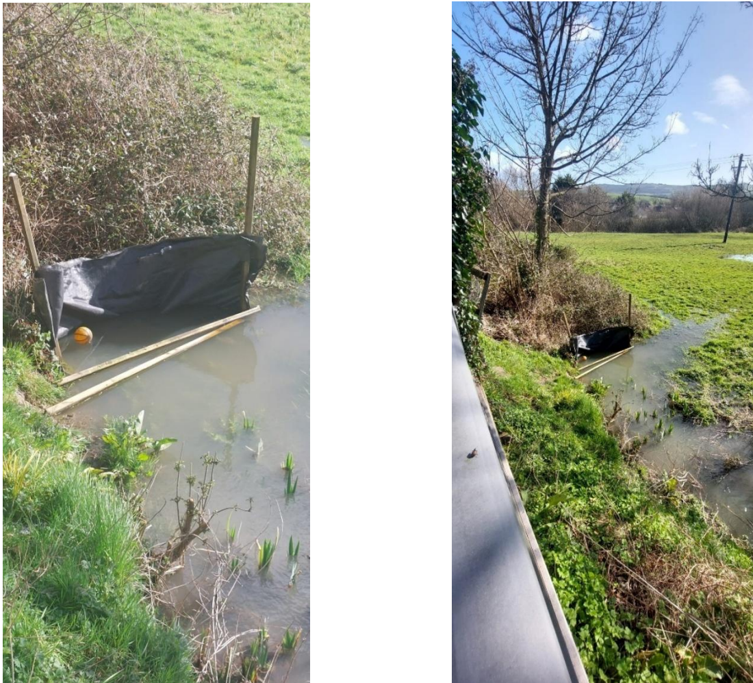
Figure 4. Small stream to the rear of Gort Na Núll in flood April 2024 with high levels of silt arises from development at Gort Na Greine.
