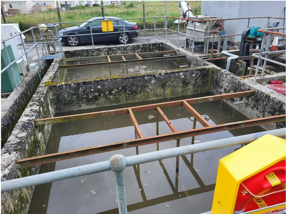
Photograph No. 3: Final clarifiers at the Lahinch WWTP which were found to be flooded due to the plant not discharging during high tides on the day off this site visit (22 nd of July 2025).
